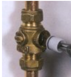
Flow restrictor installed on the sink piping.
